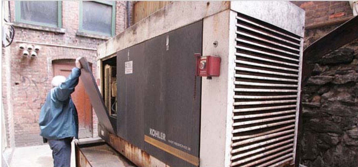
Mitch Lappin, a building superintendent at the offices of the Natural Resources Defense Council on West 20th Street, with one of the 2,236 backup generators that were counted in New York City.
